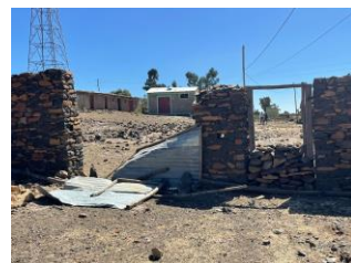
Hadnet Agricultural office entrance, network tower in background damaged © UNHCR
